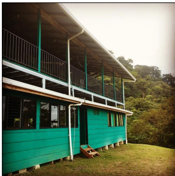
The San Gerardo station has received much-needed repairs and preventative maintenance over the past two years.
